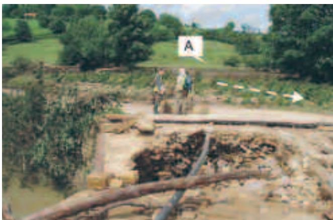
Inspecting flood damage to the bridge at Hawnby. There's a brown 'tide mark' (arrow A) of debris in the middle distance, indicating the level of the Rye floodwaters. This coincides with the floodplain (alluvium) boundary on the geological map (right). The dashed arrow indicates the direction of flow and a flattened field of small conifers.
