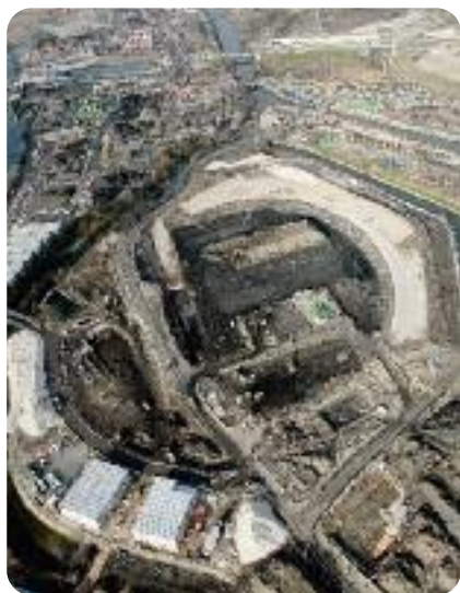
Aerial view of construction work on the main stadium for the 2012 London Olympics.
